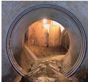
Sealing of a potable water pipe with AMEX ® -10 MONO Seal, 366 mm wide with inflating water
